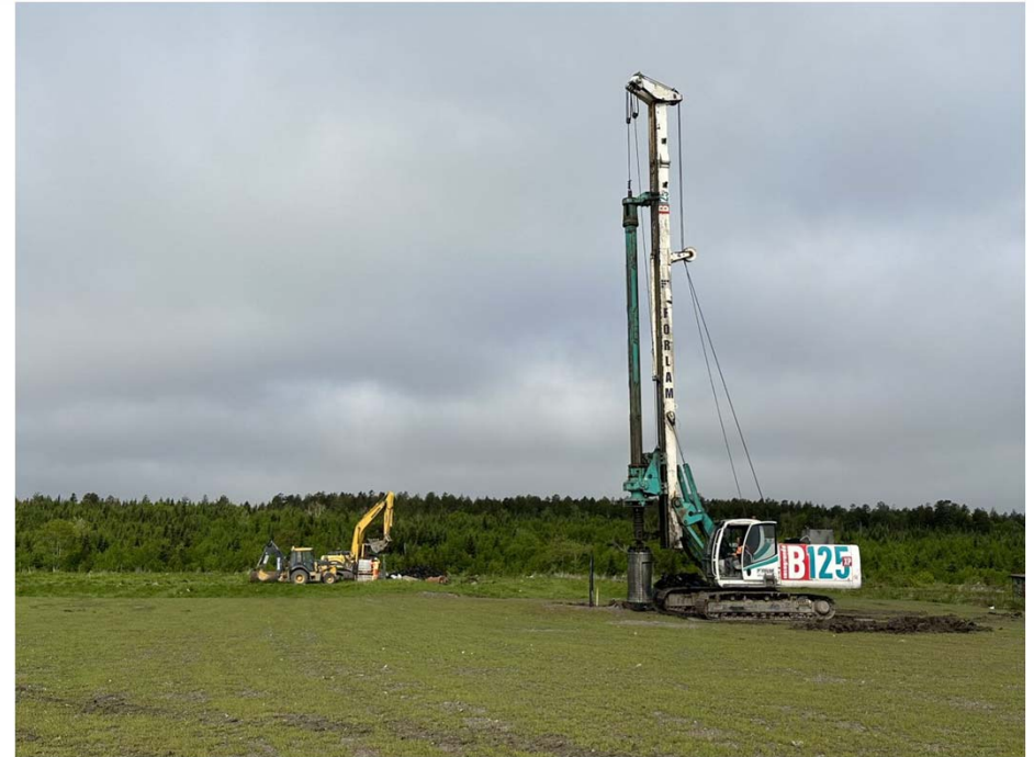
Crane Mountain Landfill Gas Well Expansion (2023)
